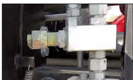
End of cable/ hook upper position automatic movement stop
